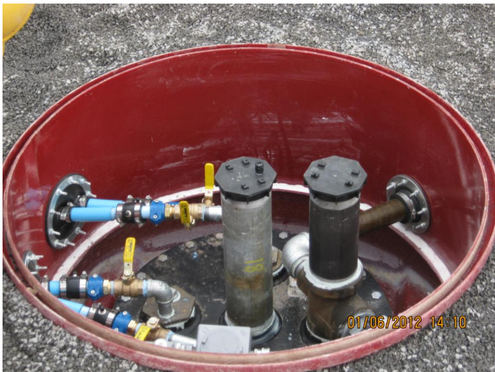
Fuel Tank Sump for New Generator
